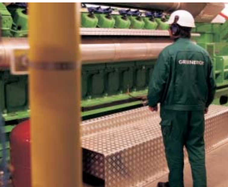
Coca-Cola HBC has identified a number of other potential sites to install all energy efficient emissions saving power generation as at the Company's plant in Hungary.
